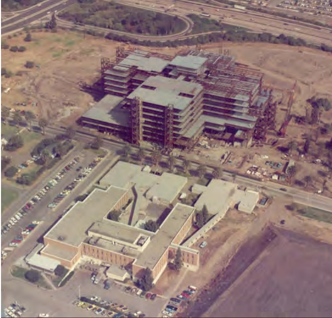
Building 304 (bottom), and Building 500 (main hospital) under construction, view northeast (VA Archives, circa 1975)
