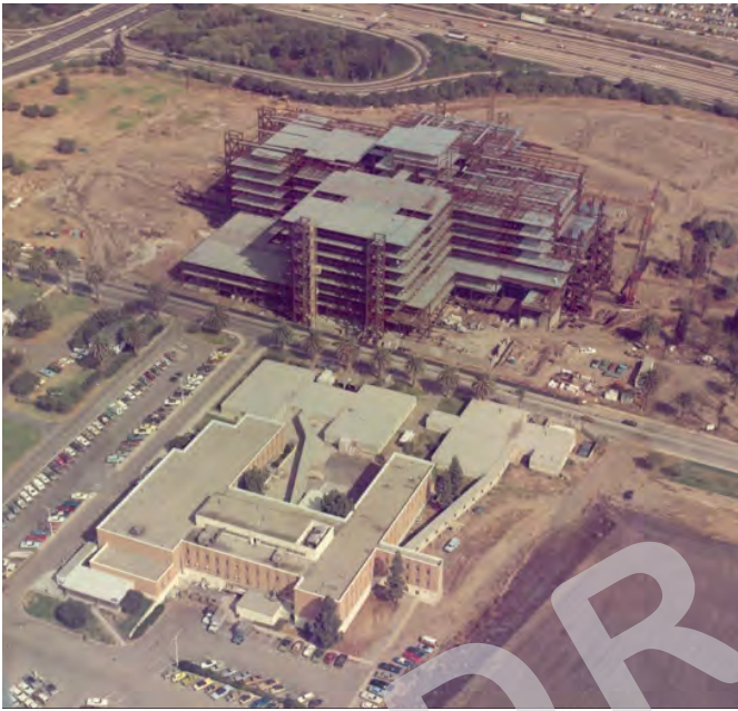
General hospital, Building 304 (bottom), and Building 500 under construction, view northeast (VA Archives, circa 1975)
